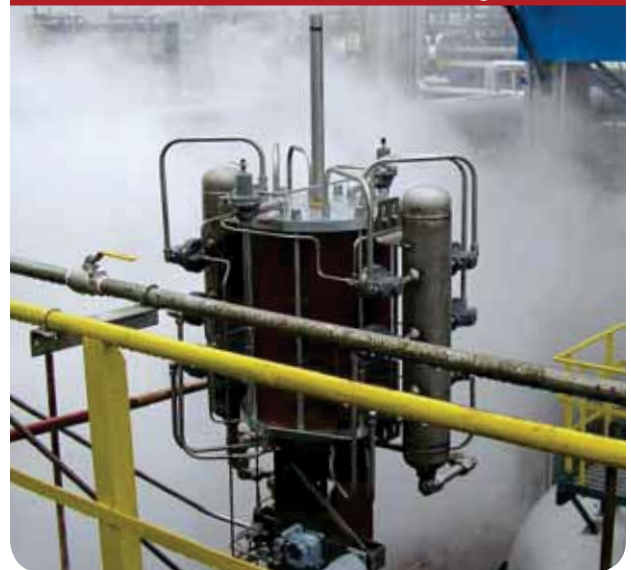
SVI II AP on steam conditioning valve
